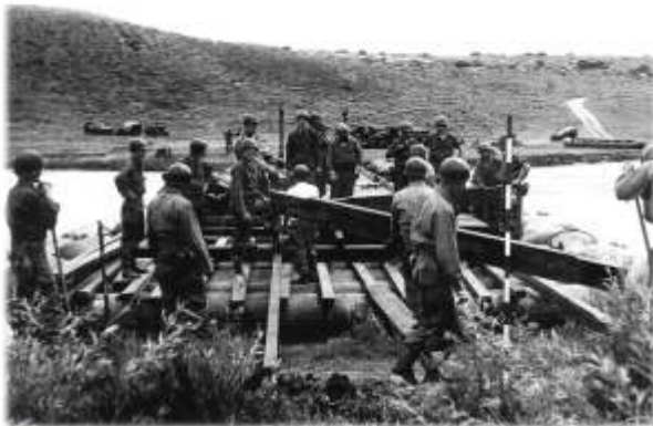
Bridge building operations were conducted from the banks of the Jordan River while under simulated enemy fire.
